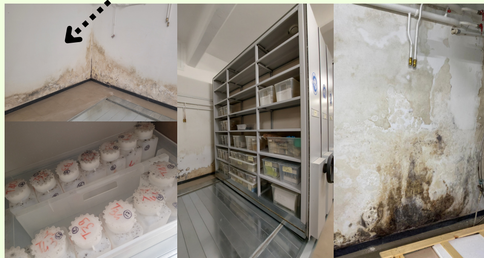
Photographs of the sampled room and objects showing clear signs of fungal contamination.
